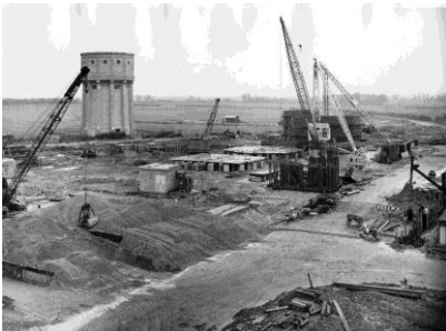
Early stages in the construction of the 8x8 tunnel in 1951, (neg RAE96212) before the water tower was moved.
